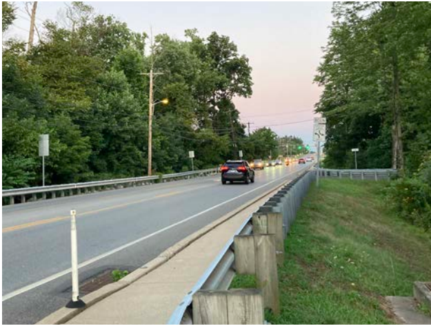
Horsham Road (S.R. 463) is an important arterial that connects the township from east to west.
