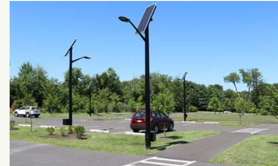
Parking lots can also be designed to incorporate other sustainable elements such as the solar-powered parking lots lights at the Montgomery Township Community Center.
