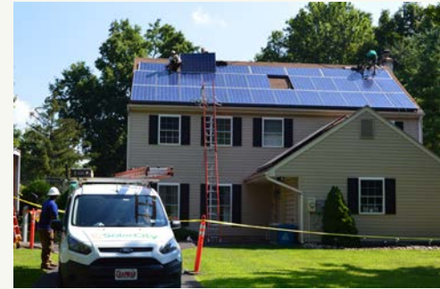
Example of solar photovoltaic (PV) panels installed on a single-family residential home in Horsham Township.
