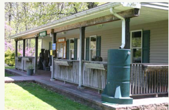
Rain barrels allow rain water from a building's roof to be collected on-site and slowly discharged after the rain storm to reduce the peak flow of stormwater in nearby streams that can occur during a storm."
