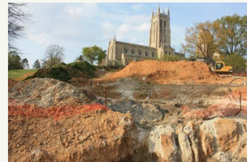
Example of an underground geothermal energy system being installed on a church property in Bryn Athyn Borough.
