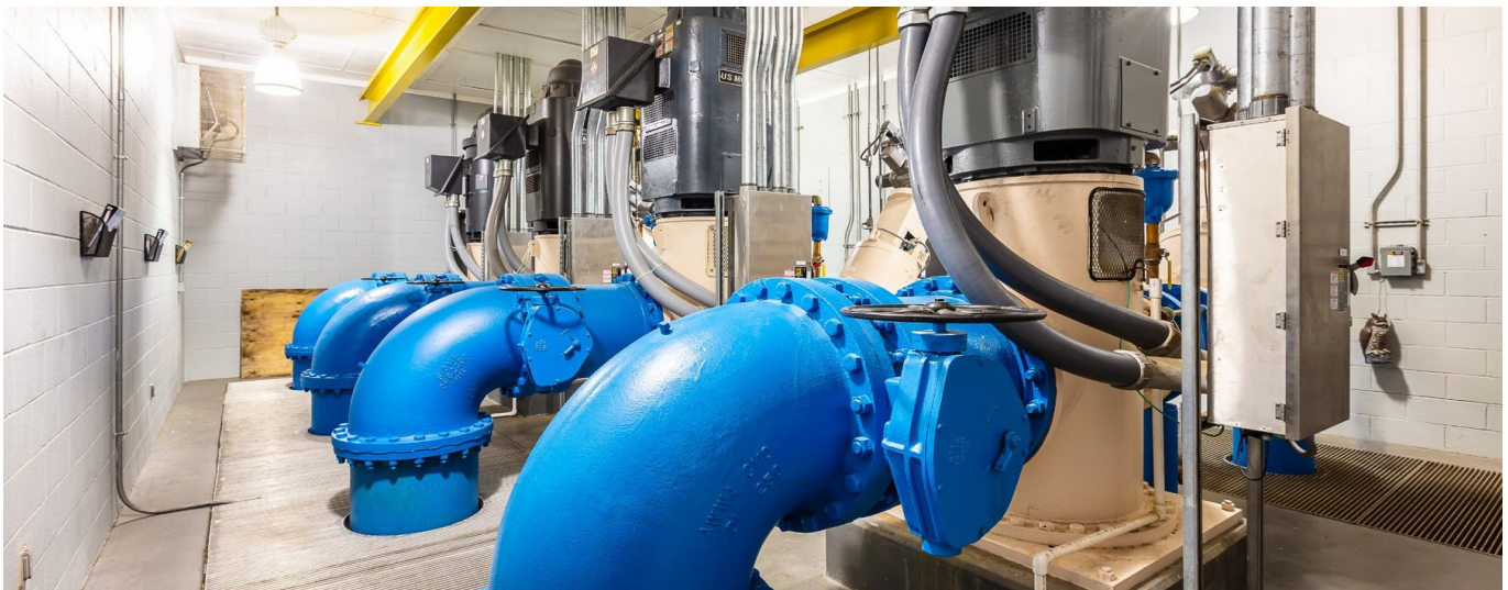
MVUD pump station infrastructure, including four 600 HP motors, helps move water through the District's distribution system.
