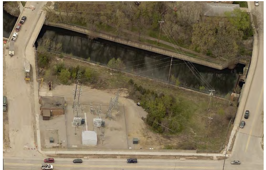
Birds-eye view of the Interstate Power (Alliant Energy) land on the south side of Willow Creek, looking north
