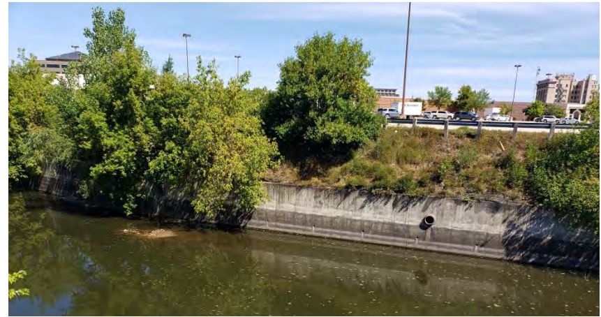
North side of Willow Creek, below the Mall parking lot, west of the US 65 North-bound Bridge
